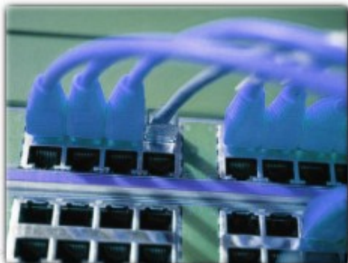
Cable and switch
